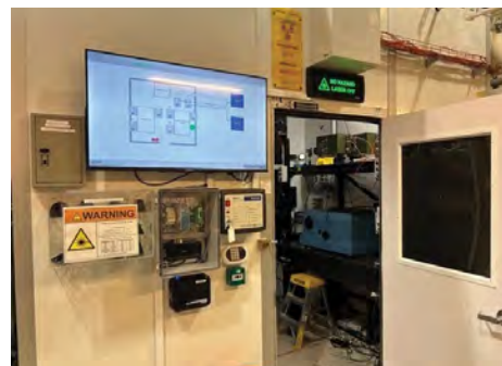
Figure 6. New laser interlock system. Image on the screen shows whether any of the lasers are interlocked and whether the room is safe to enter.
