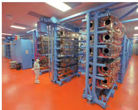
Figure 1. Photograph of OMEGA 60-beam UV laser beamlines showing the power amplifier clusters. The final amplifiers on OMEGA are 20-cm diameter Nd:glass disk amplifiers.
