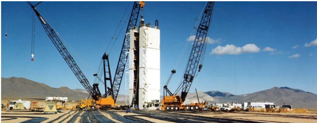
Figure 37. Temporary structure holding test canister for final assembly of nuclear test. Coaxial cables to transmit measurements lie on the ground. Crane holds canister over hole.
